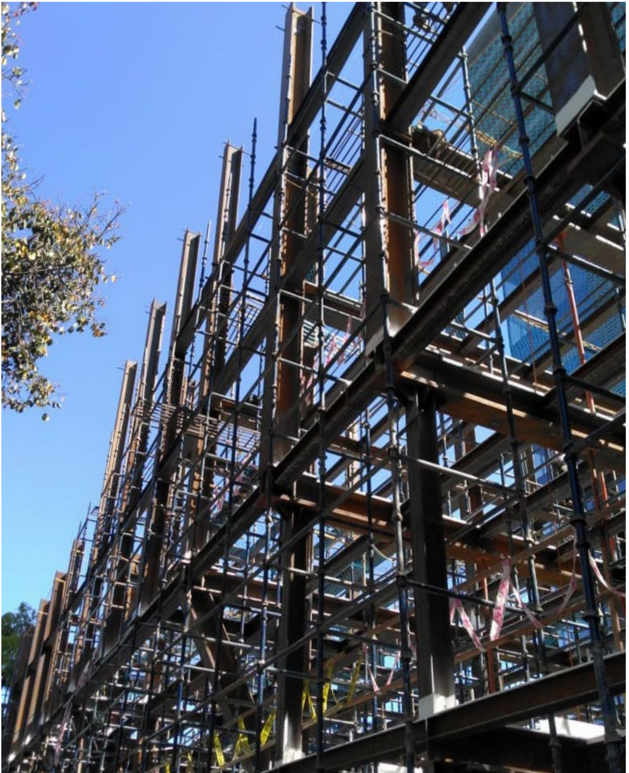
As of date, the structural steel beams and the erection of columns up to the third floor is complete. The fourth floor beams are still under construction.
